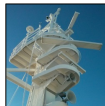
Rutter radar antenna (center)
